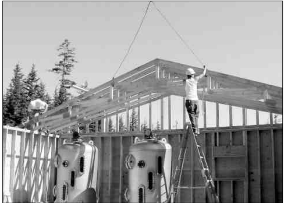
Carpenters place roof trusses onto the walls of Tatitlek's new water treatment plant.
