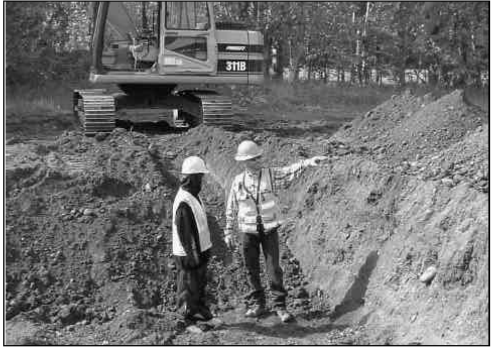
NIT Trainer Gene Peoples (right) instructs Vernon Madros Jr. from Nulato (left) on proper excavating techniques at the construction skills training in Palmer.
