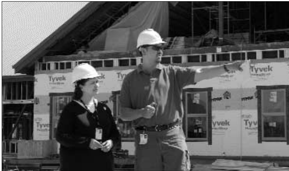
Rachael Askren, Service Unit Director of the Annette Island Service Unit, and Butch Hayward, AISU Project Manager, monitor progress on the new Health Center in Metlakatla.
