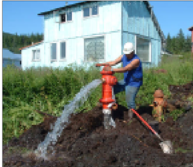
Equipment Operator Gusty Wassillie tests a newly installed fire hydrant before final grading in Tatitlek, Alaska. In recognition for this project's contributions to diversity, the American Public Works Association awarded DEHE the Diversity Exemplary Practices Award in September 2004.
