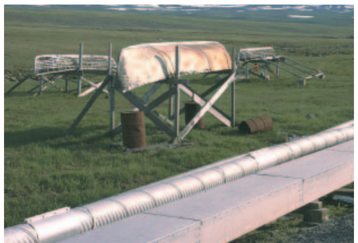
In the northwest Alaska village of Savoonga, umiaks rest near the utilidor that shelters almost three miles of piping for water and waste-water. The project serves about 650 residents. Modern sanitation has greatly improved quality of life for Savoonga residents.
