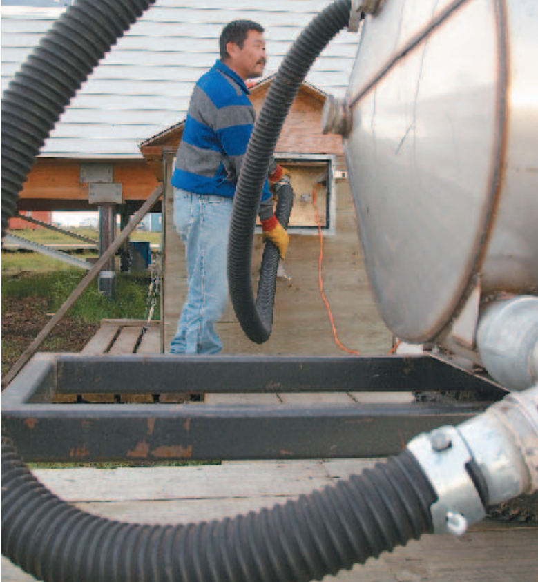
Nunapitchuk Water and Sewer Operator Edward Andrew uses a vacuum truck to empty a home's septic storage tank. Such advances in clean water and sanitation systems have made death from gastrointestinal disease a thing of the past.
