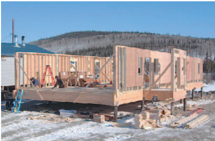
Tetlin's new 2,000-square foot health clinic, funded by the Denali Commission and designed and built by the Alaska Native Tribal Health Consortium, will provide health services to 130 residents. The clinic was completed in November 2003.
