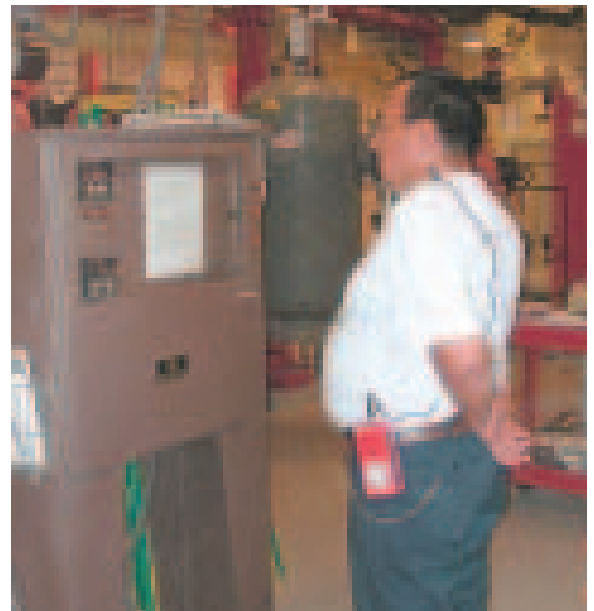
Using a dosimeter, Lead Utility Systems Operator Roman Albert measures noise levels in the boiler room at Yukon-Kuskokwim Delta Regional Hospital.
