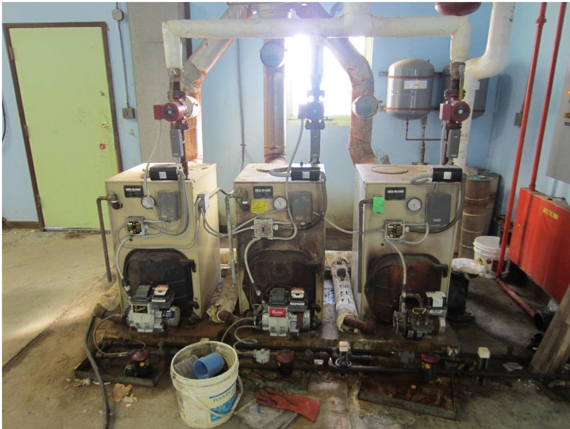
Figure 5: Boilers in the upper pump house.
