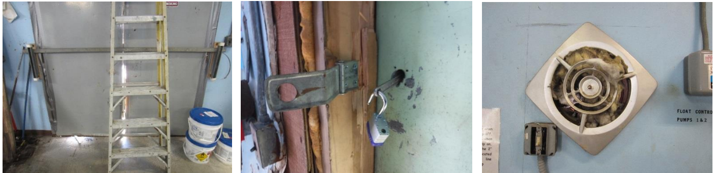
Figure 10: From left to right: Air leakage around side doors, current locking mechanism on front door, old vent fan open to exterior.
