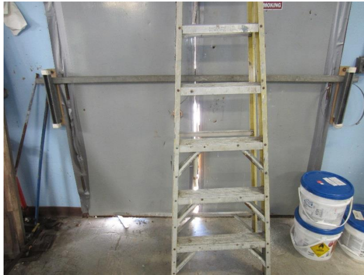
Figure 4: Air leakage visible around side doors.
