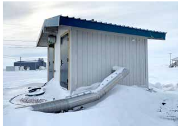
Savoonga Lift Station
