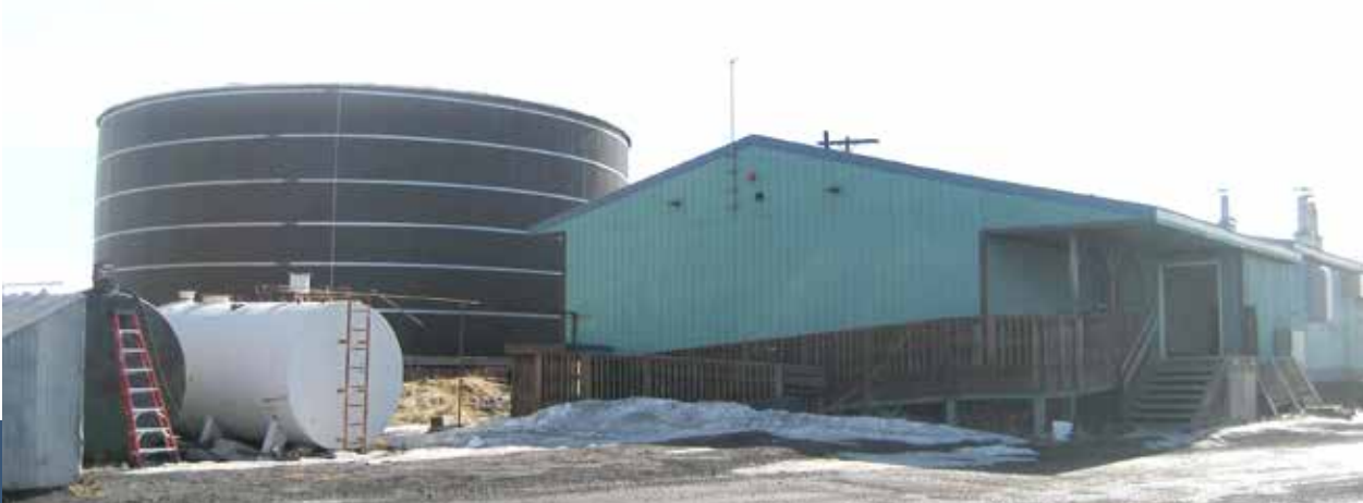
St. Michael's Water Treatment Plant
