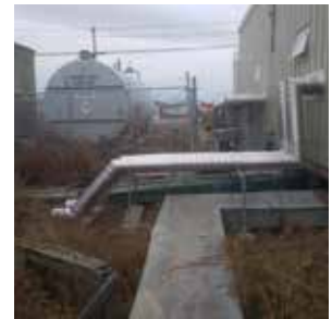
Noorvik Heat Recovery Expansion
