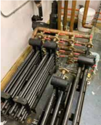
Saint Michael Heat Exchangers
