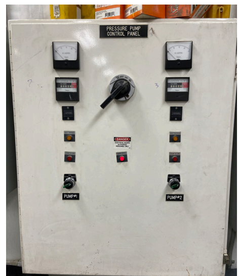
Kiana's New Control Panel
