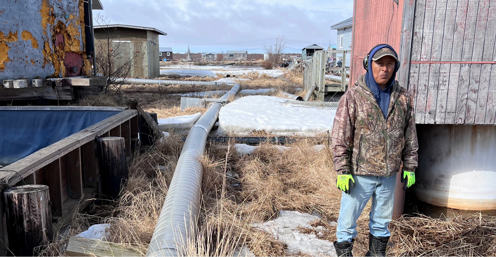
Kotlik Washeteria Water and Sewer Connection
