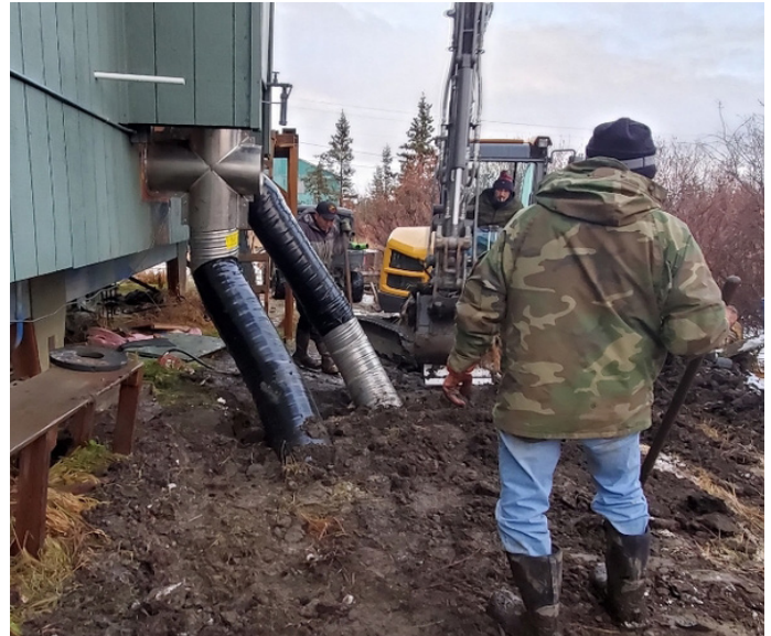
Kiana Water and Sewer Flex Connections
