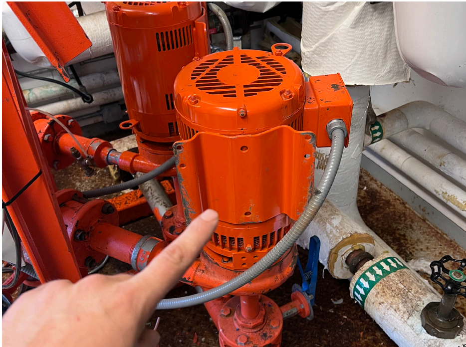
Scammon Bay Pressure Pump Station
