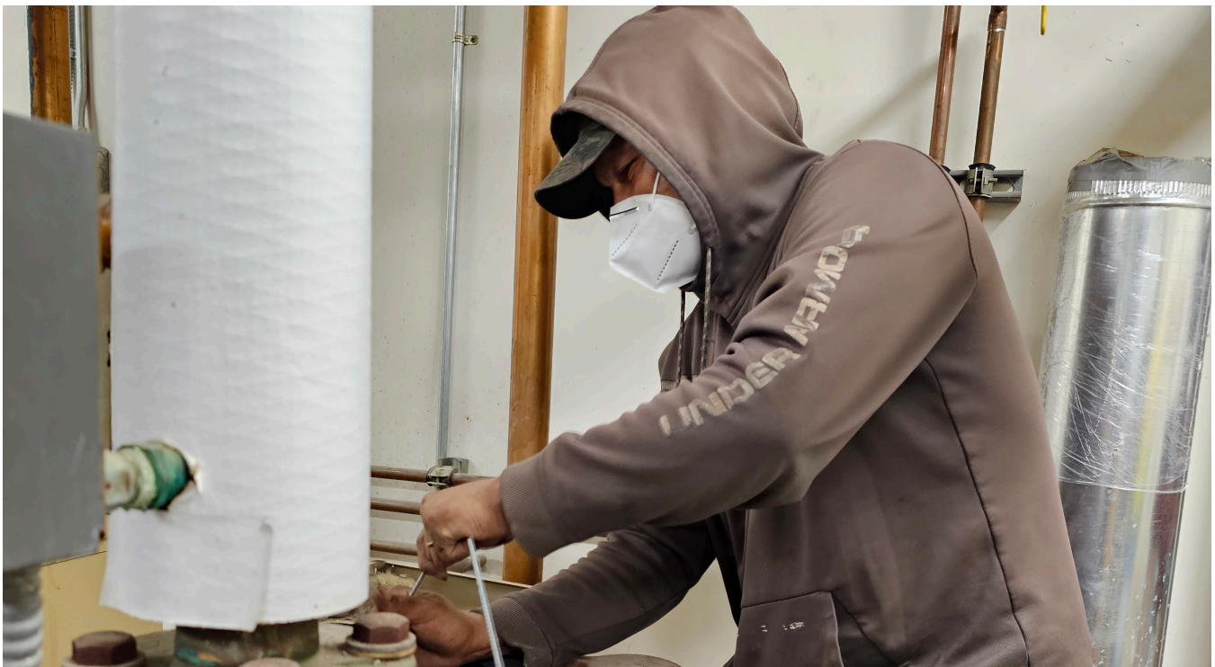
Adolph Pleasant, Quinhagak water plant operator, at ARWA training
