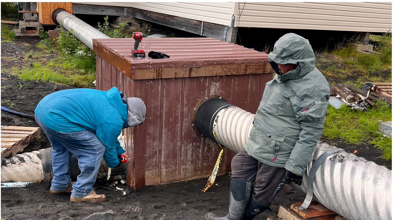
Saint Michael Duplex Service Connection
